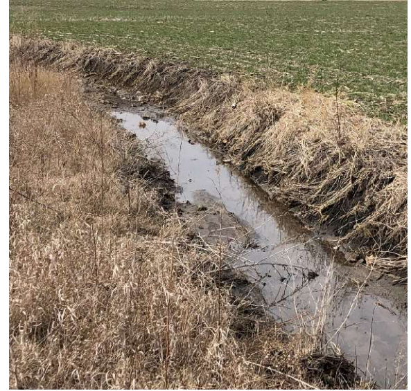
Pictured: Gully Found in Will County
